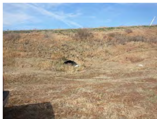
Photo 8 - 24" CMP along I-15 south of Nichols Road
